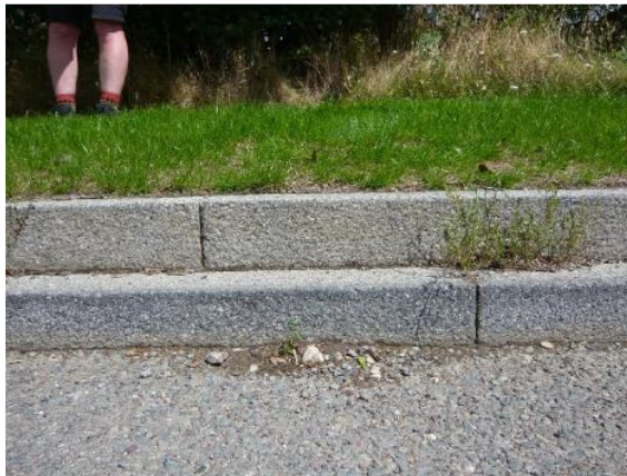
Observed difference between carriageway and footway level
